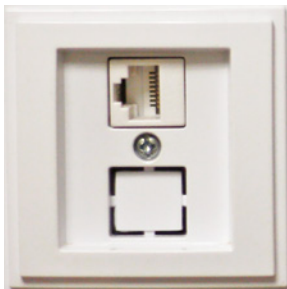
FIGURE 16.5 A network connection in a wall
